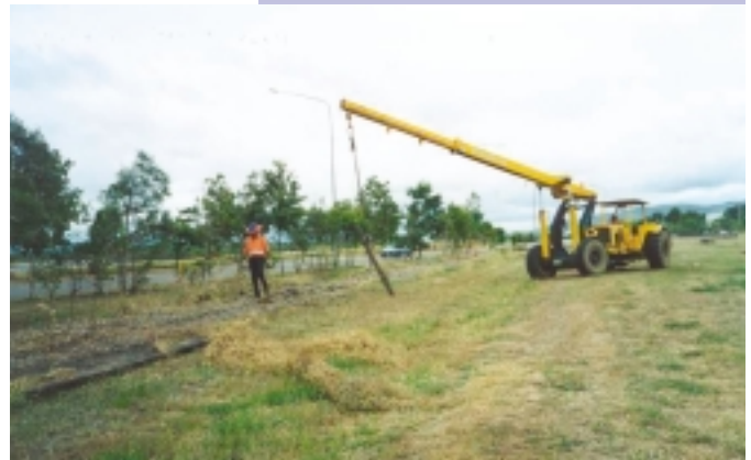
The removal of the old rail line was undertaken in such a manner to avoid noise and dust problems for South Townsville residents.
