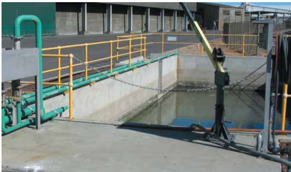
Photograph showing one of the concrete containment sumps and associated water treatment and pumping equipment.
