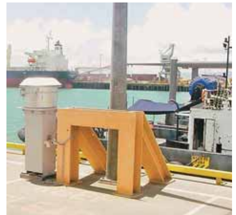
Figure 3. PM10 High Volume Air Sampler at Berth 9 with Berth 3 in the background.
